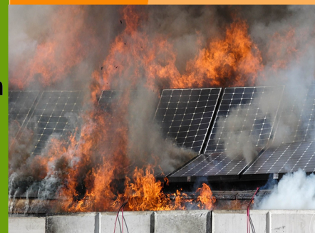
(3) Solar PV panels fire incident.
