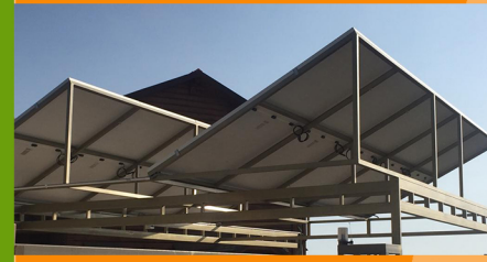
(1) Roof mounted PV panels frame
