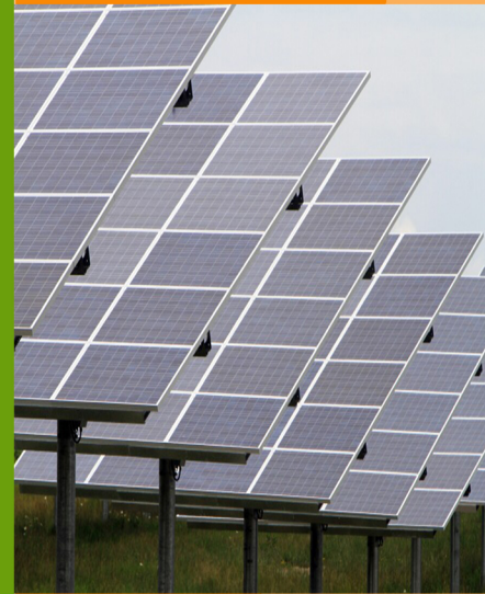
(2) PV panels oriented to south direction
